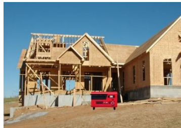
Construction Power Backup
