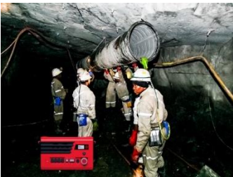
Mining Power Backup
